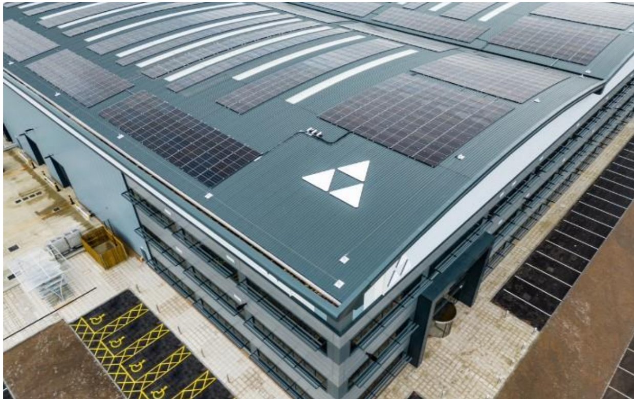
Fig 68. Illustrative example of a PV installation on the roof.
